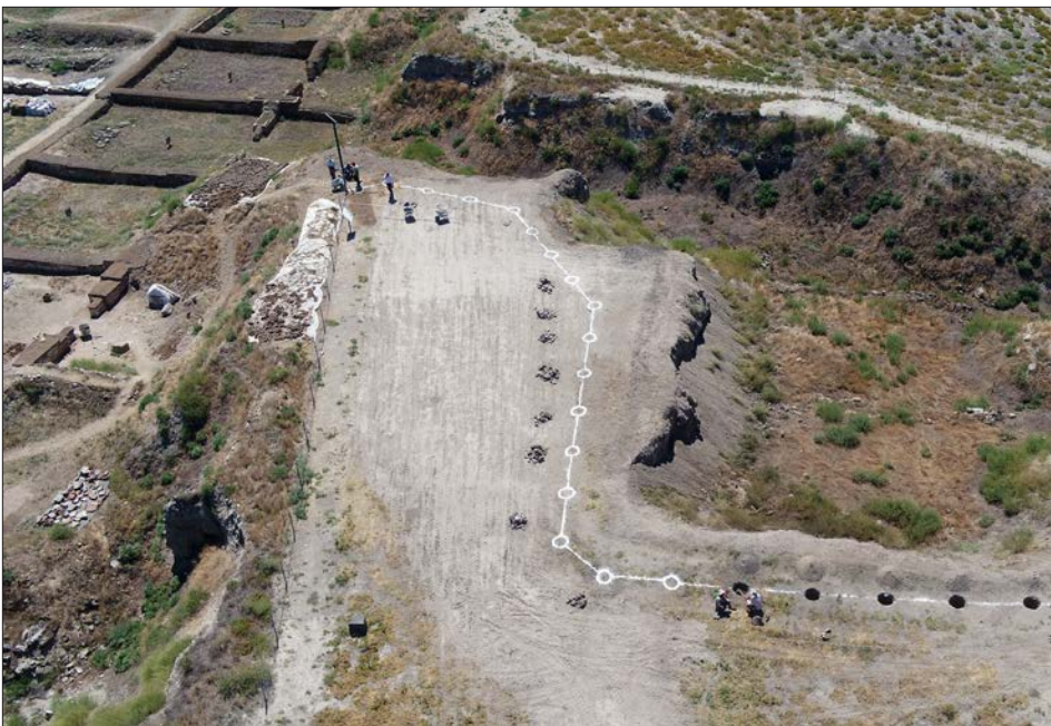
Figure 9: Installation of the new fence on the Visitor Circuit, looking south. The Terrace Building is at upper left. Photo by Ali Can Kırcaali and Zekeriya Utğu.
