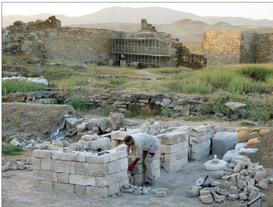
Figure 6: The new stone encasement around the damaged walls of Megaron 3, with the citadel's East Gate at top, looking southeast. Photo by Elisa Del Bono.
