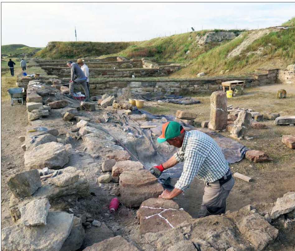
Figure 7: Conservation of the damaged walls of unit 7 of the Terrace Building (TB-7), looking southeast. The new security camera is the tall, slender looking object visible on the skyline at left. Photo by Elisa Del Bono.
