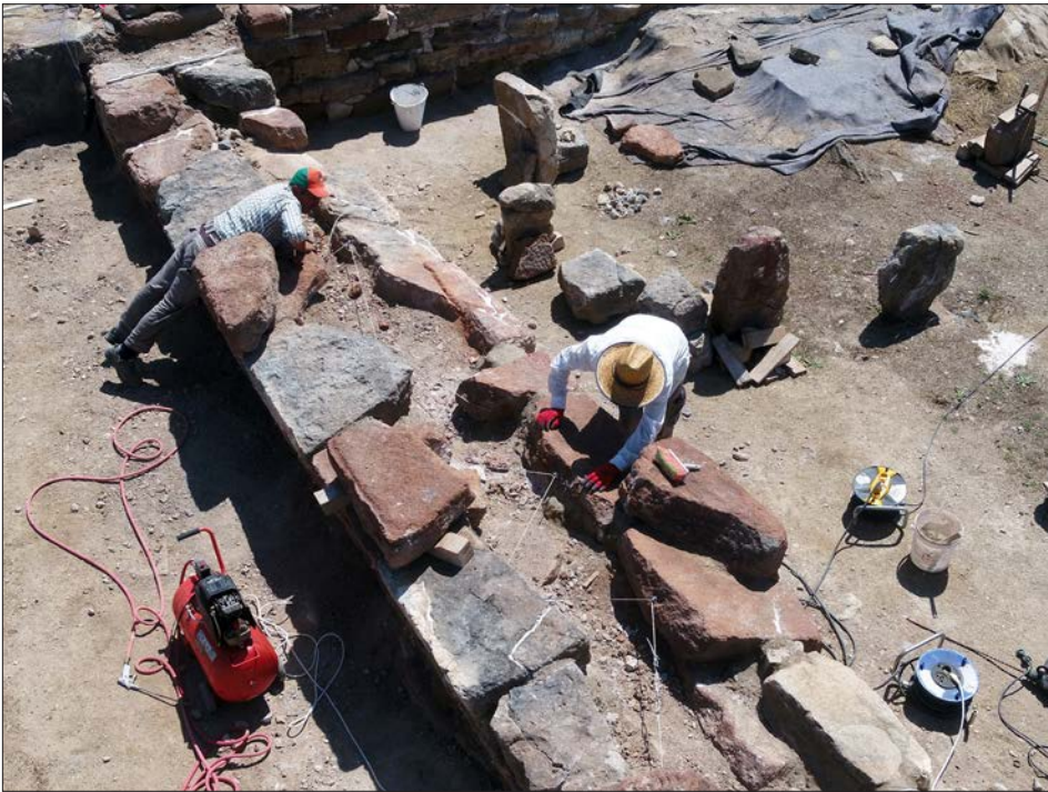
Figure 8: Conservation of the damaged walls of unit 7 of the Terrace Building (TB-7), looking southeast: insertion of steel cables through the core of the wall to secure the facing stones. Photo by Elisa Del Bono.
