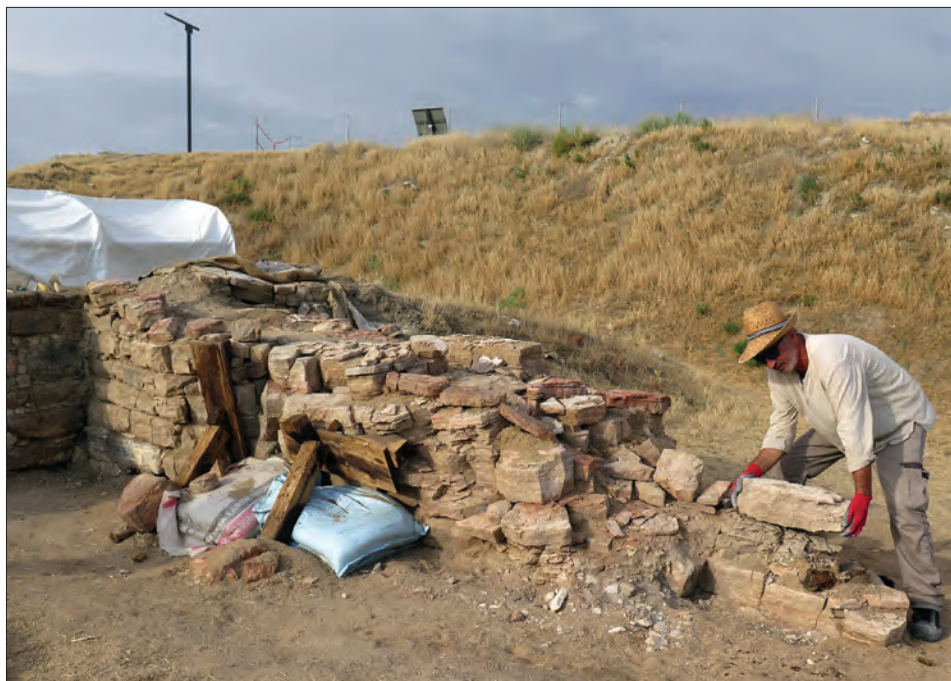
Figure 7: The damaged partition wall of the Terrace Building's TB-8 unit (9th century BCE), before conservation, with Angelo Lanza beginning the work. Photo by Elisa Del Bono.
